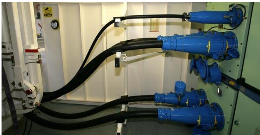
Figure 14. Ship connection panel with HVSC power cables attached
